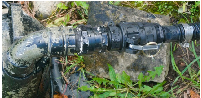
Tim bought a 1.25 inch quick disconnect for the connection between the pump and the hose.
